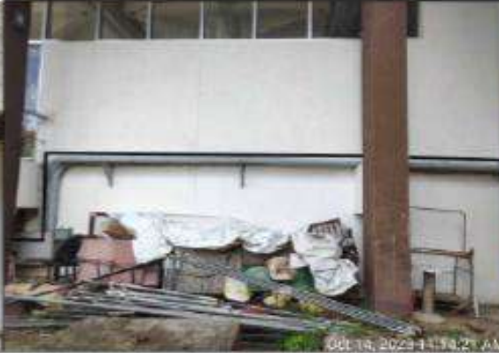
Main Electrical Room
