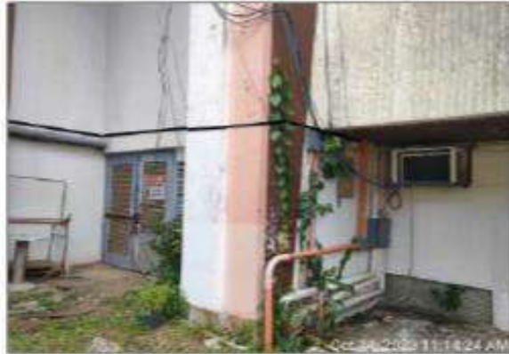
Main Electrical Room, & PABX Room
